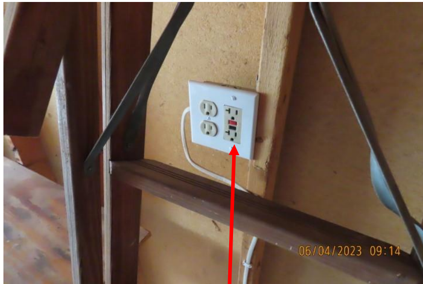
GFCI tested faulty
