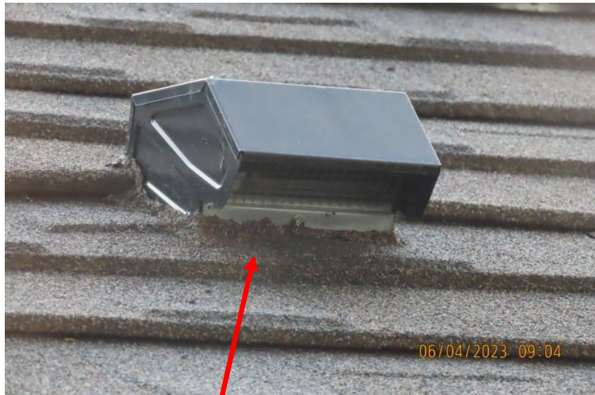
Flashing is incomplete
