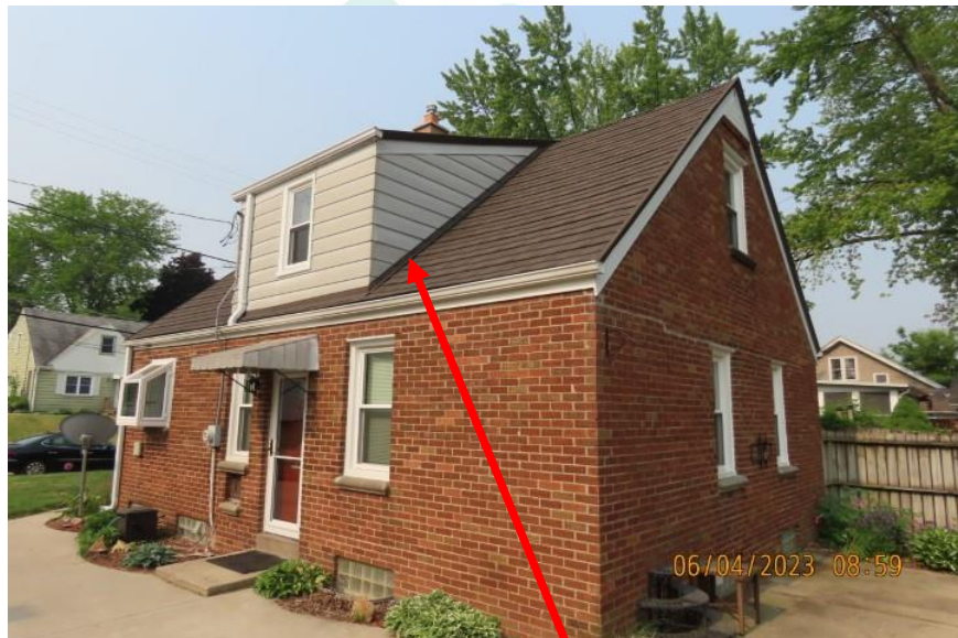
Flashings are incomplete
