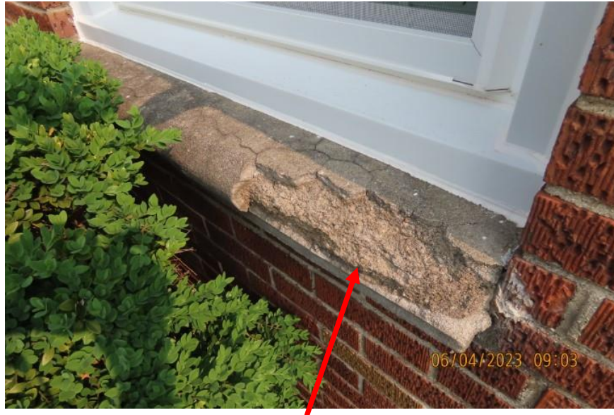
Concrete sills need repair
