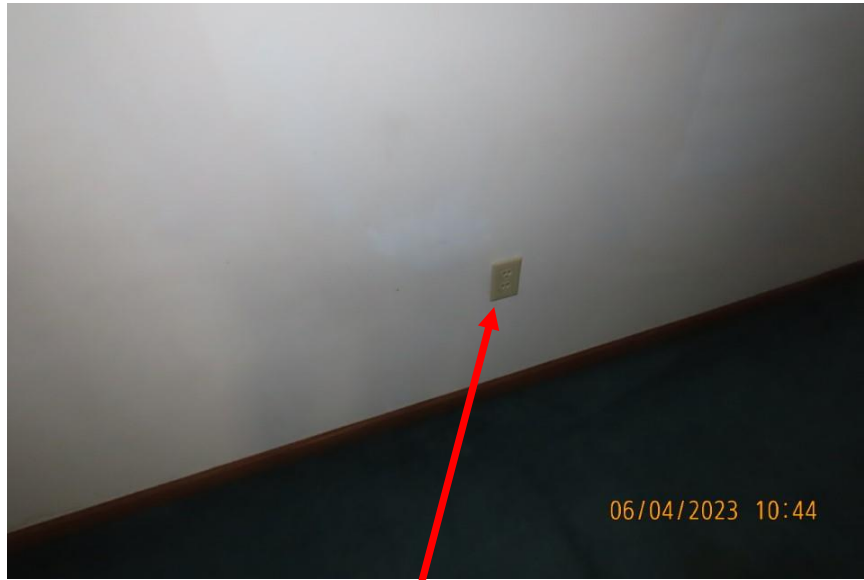
Loose outlets need to be secured
