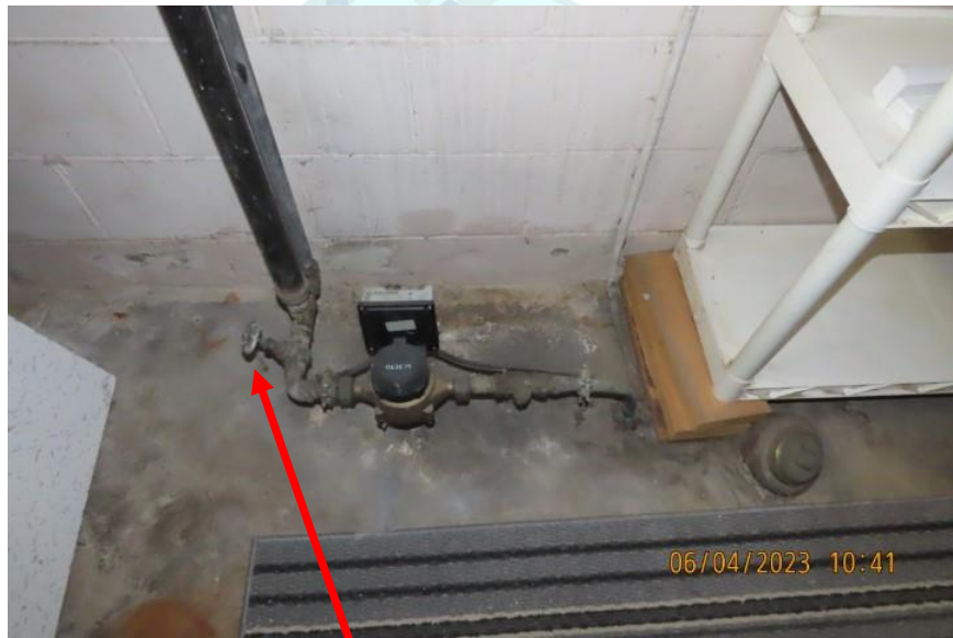
Main Water Shut Off
