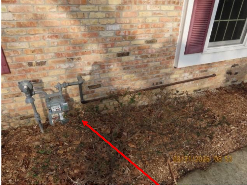
main gas shut off
