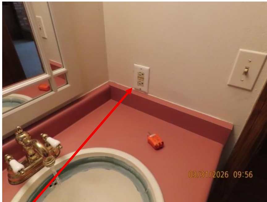
The first floor bathroom GFCI did not trip upon testing
