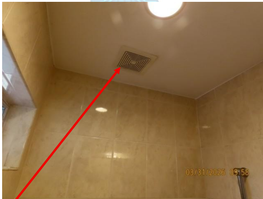
bath fans within the shower cavities must be protected by a GFCI
