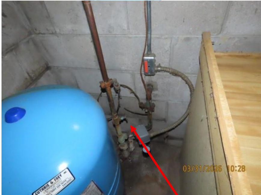
main water shut off
